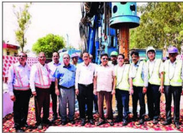
Piling work is done to build foundation of structures for building elevated viaducts
