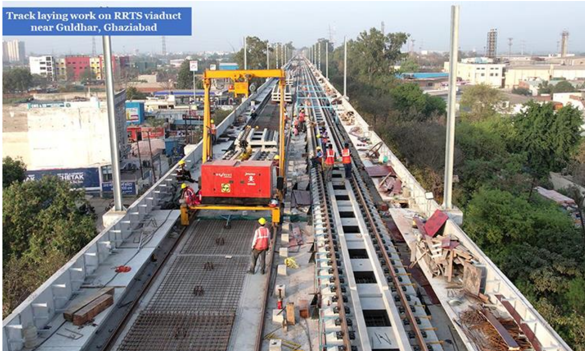
Credit: NCRTC – Track laying work on a RRTS viaduct section near Guldhar, Ghaziabad.
