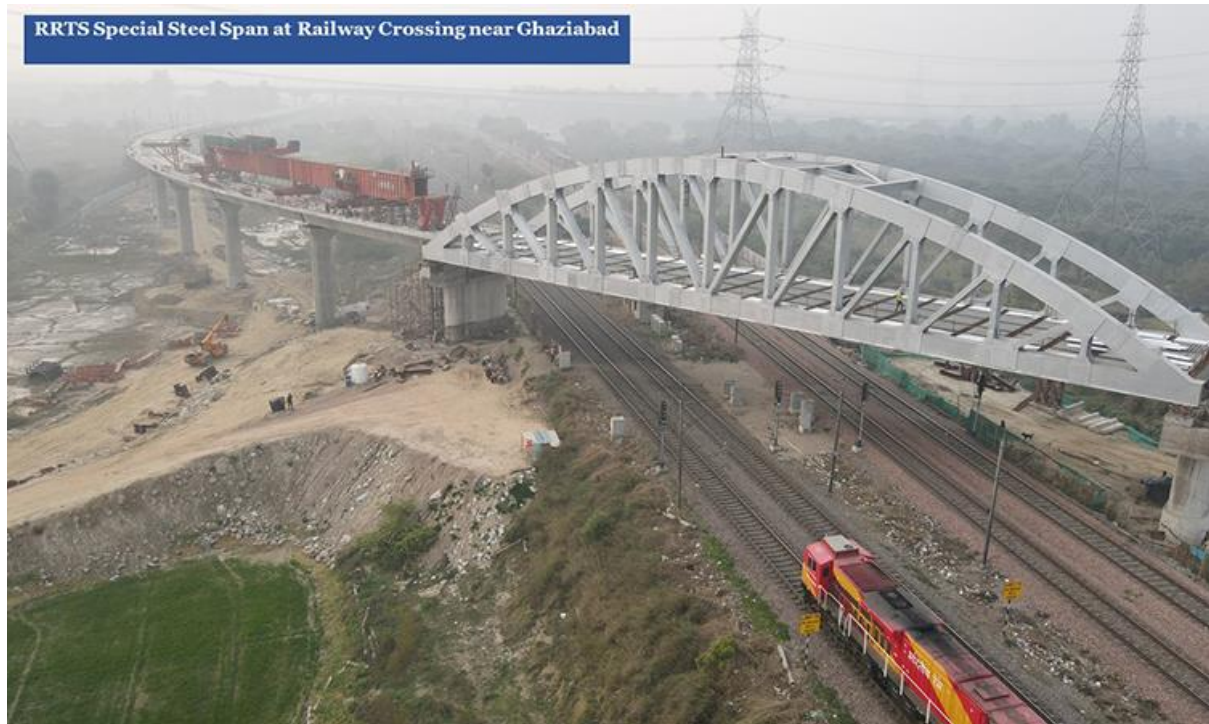
Credit: NCRTC – Steel bridge construction for the RRTS network crossing over the railway near Ghaziabad.
