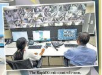
The RapidX train control room.
