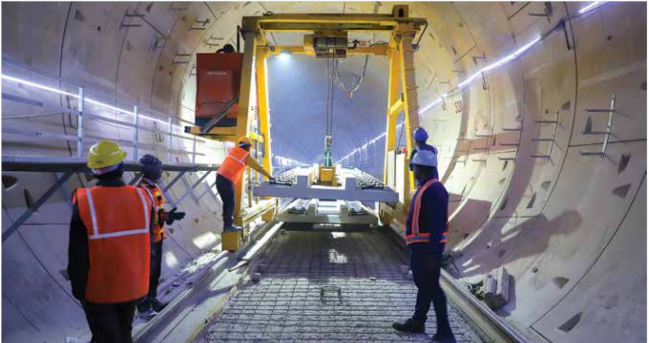
Work in Meerut section of the Delhi-Meerut RRTS corridor in advance stages
